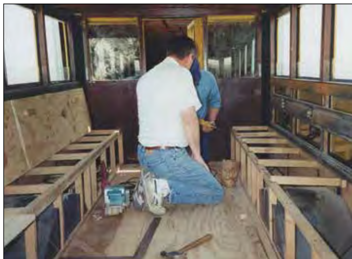
Pat Heitkamp, Will Prenger's son-in-law and the bus's current owner, and Prenger install seats in 1999.
